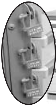
Close-up of system
